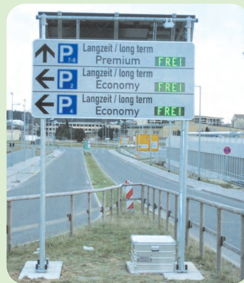
Electric parking guidance system
